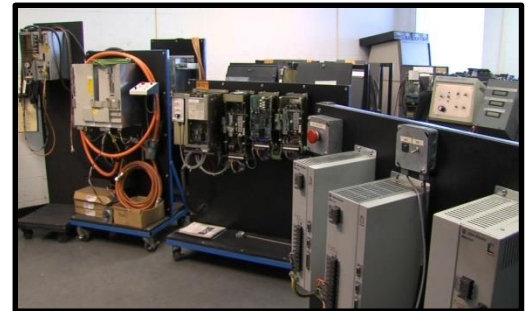
Dedicated Test Stands
